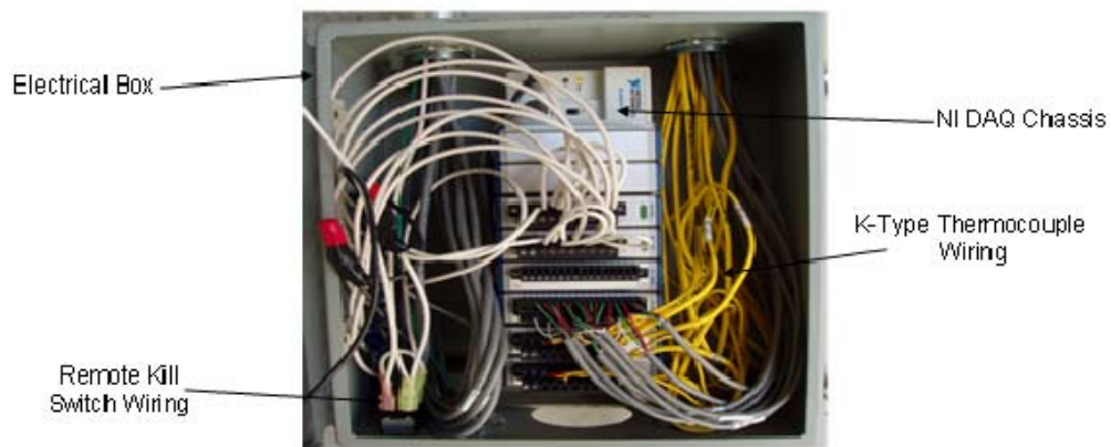
Figure 26. Electrical box internals
