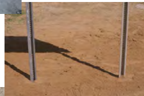
Fracturing Sign Support
