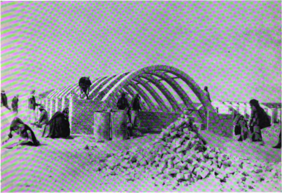
PLATE XXXVI. Iraq. A Surgical Ward of 61 British General Hospital, Shuiaba, under construction. Built of crude bricks, the arches have no keystone. They are covered with straw and lined with plaster.
