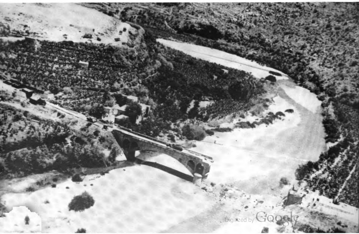
36. The broken bridge at the mouth of the river Damour.
