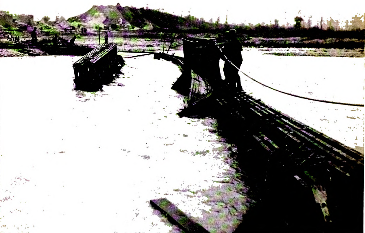
20. Italy. Flood. A bridge over the River Sangro, wrecked.
