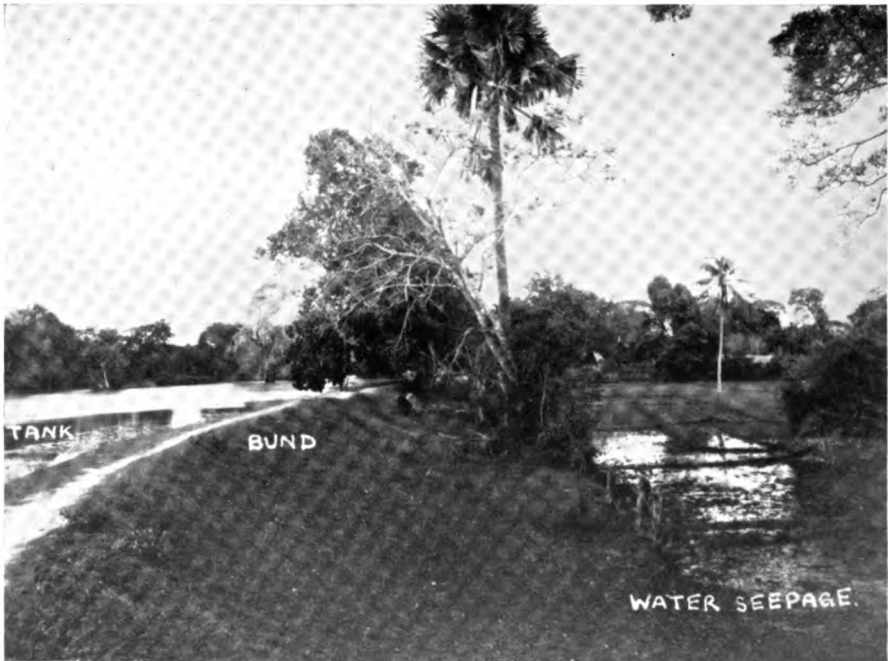
PLATE XLIV. Man-made malarial hazard. Water seepage from a storage tank— a serious malaria risk.
