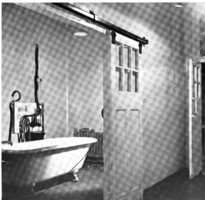
PLATE XXXVIII. Saline bath installed in special bathroom with sliding doors for easy access of stretchers.
