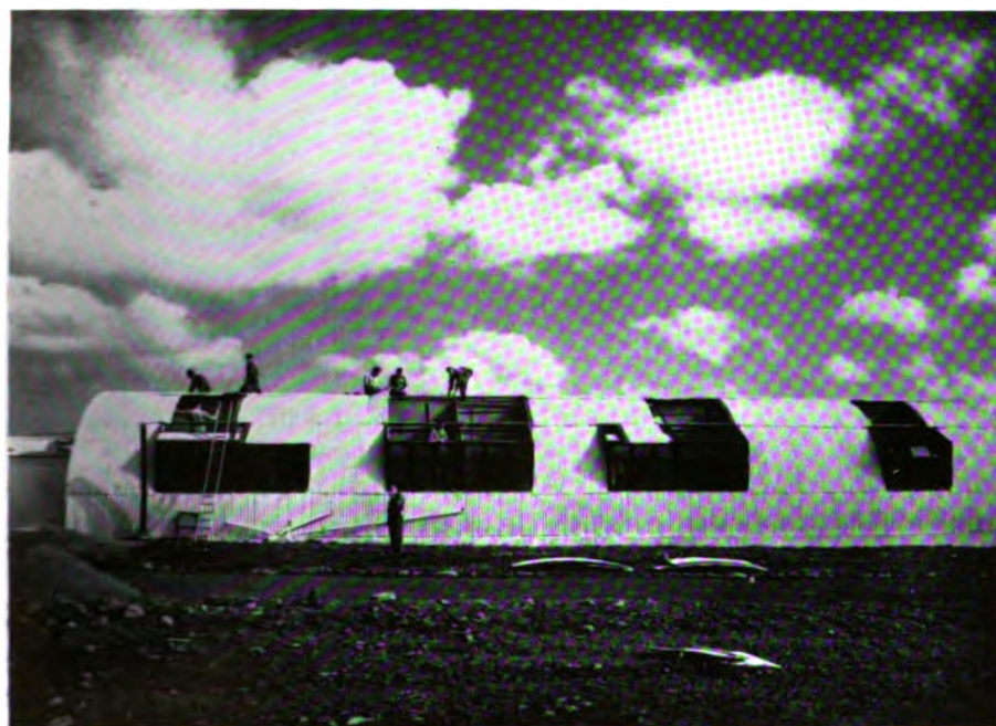
PLATE XXVI: Repairs being effected to R.A.F. Hospital, Lagens, after the Hurricane and Rainstorm in October 1944
