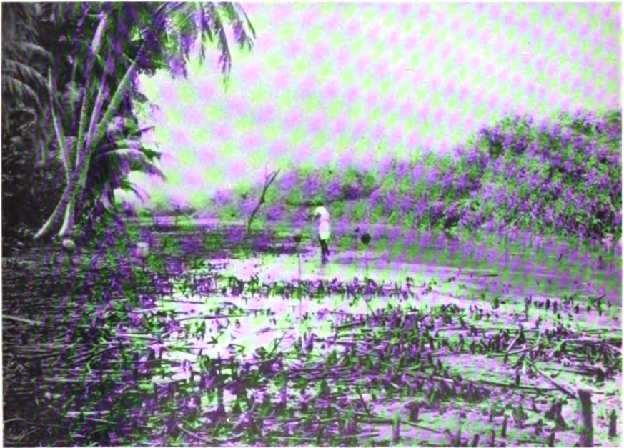
PLATE XXXIII : Swamp after preliminary clearance. Staves topped with coconut shells mark future drainage channels
