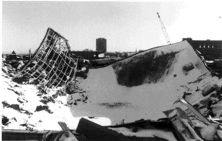
Fig. 2. Collapse of the Hartford Civic Arena roof following a winter storm with snow and freezing rain (January 18, 1978).
